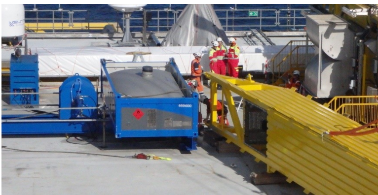
Picture: Winch frame
