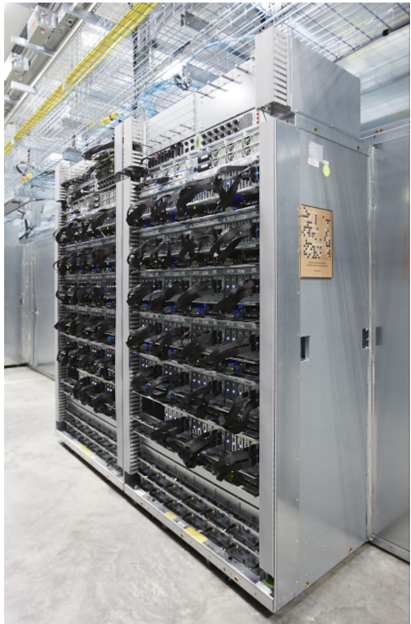
A custom rack in a Google data center packed with Tensor Processing Unit hardware for machine learning. (Photo: Google)
