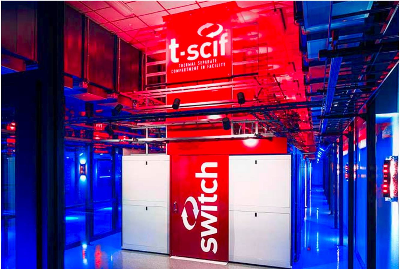
A TSCIF aisle containment system inside the SUPERNAP campus in Las Vegas. (Photo: Switch)
