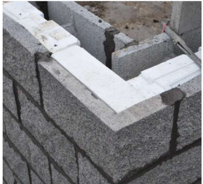
Corner with L-shaped fitting cut from CMU and soap. The face shell of the HI-R-H unit to the right can be cut as needed to accommodate horizontal reinforcement
