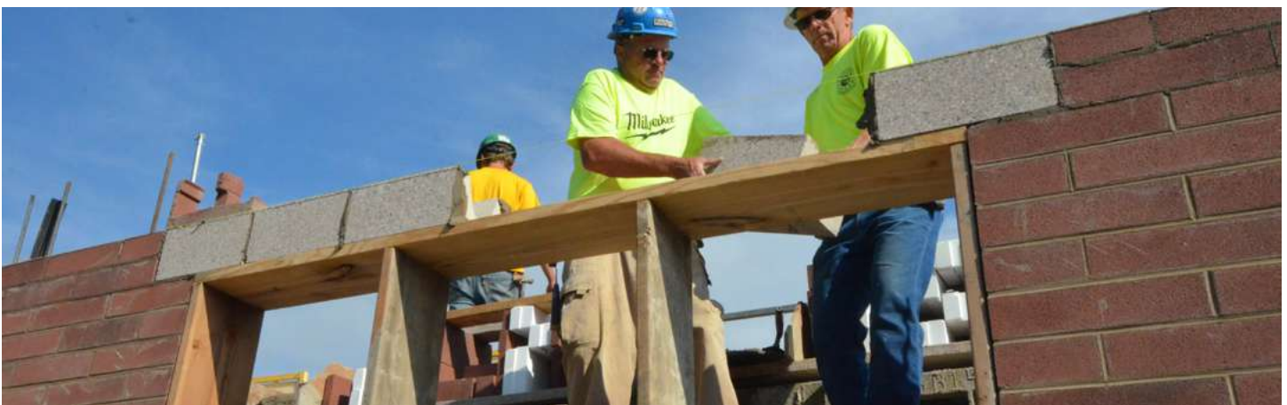
Traditional masonry lintel installation using a form (this lintel is not insulated)
