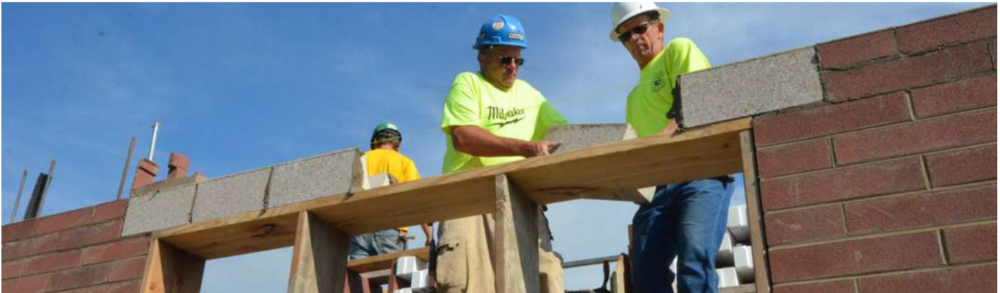
Traditional masonry lintel installation using a form (this lintel is not insulated)
