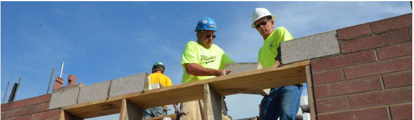
Traditional masonry lintel installation using a form (this lintel is not insulated)
