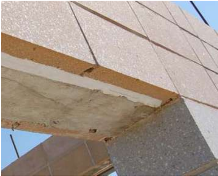
HI-R reinforced as lintel after grout has cured and wood forms have been removed
