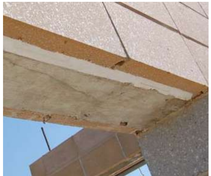
HI-R unit reinforced as lintel after grout has cured and wood forms have been removed
