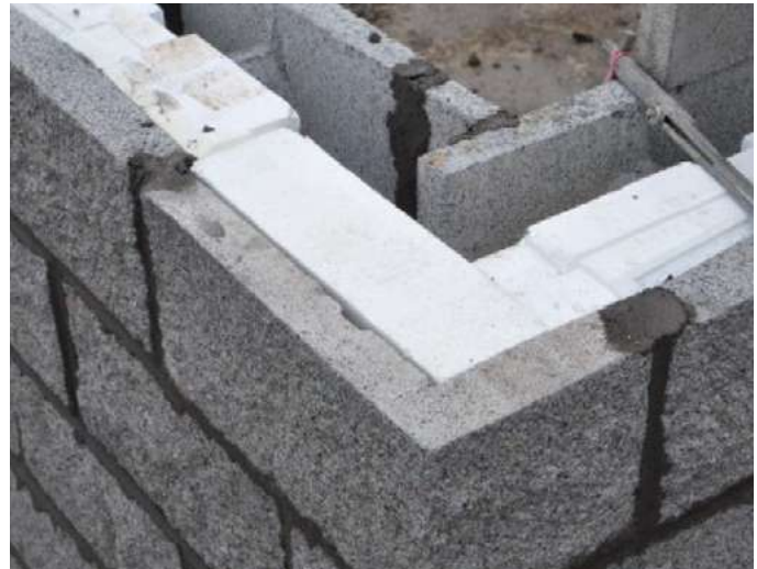
Corner with L-shaped fitting cut from CMU and soap. The HI-R-H unit to right's face shell can be cut as needed. This detail can be used with both HI-R and HI-R-H units as well as the Half High versions of each
