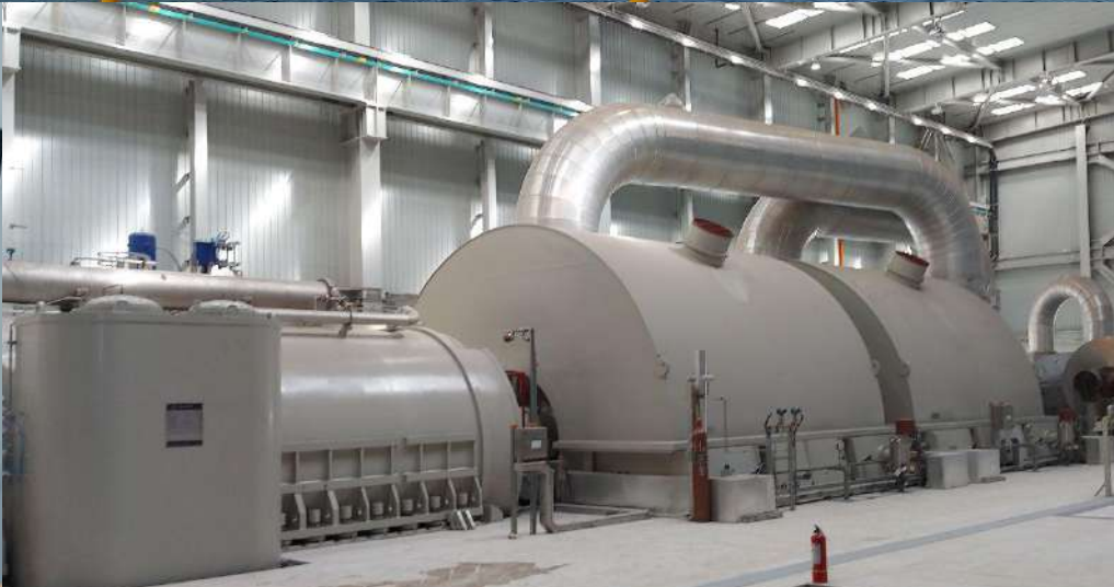
Unit 1 Steam Turbine Generator
