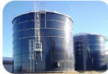
Increased water storage capacity
