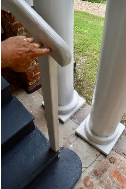
Fig. 10. Loose wooden handrail - south elevation, west side.
