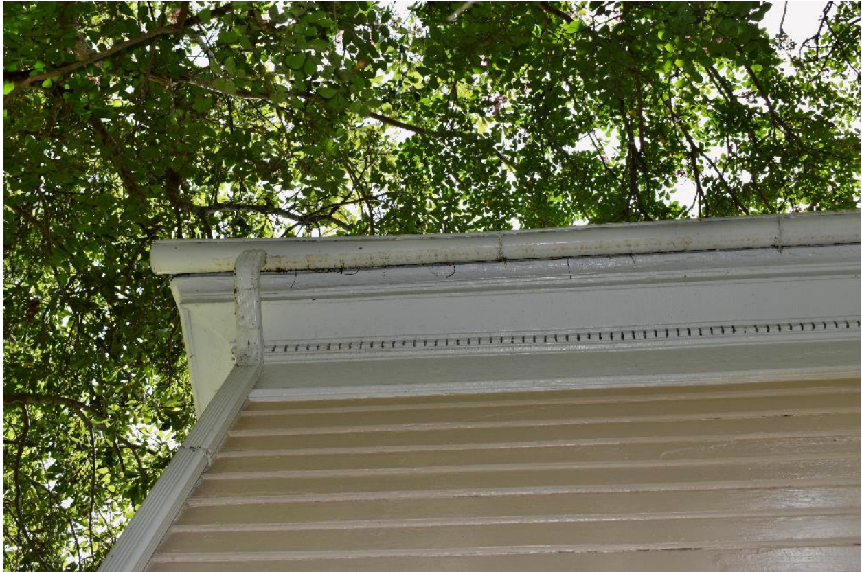
Fig. 18. Overhanging tree limbs – northwest side of library wing
