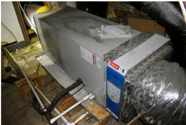
Fig. 14. Attic HVAC unit. system.
