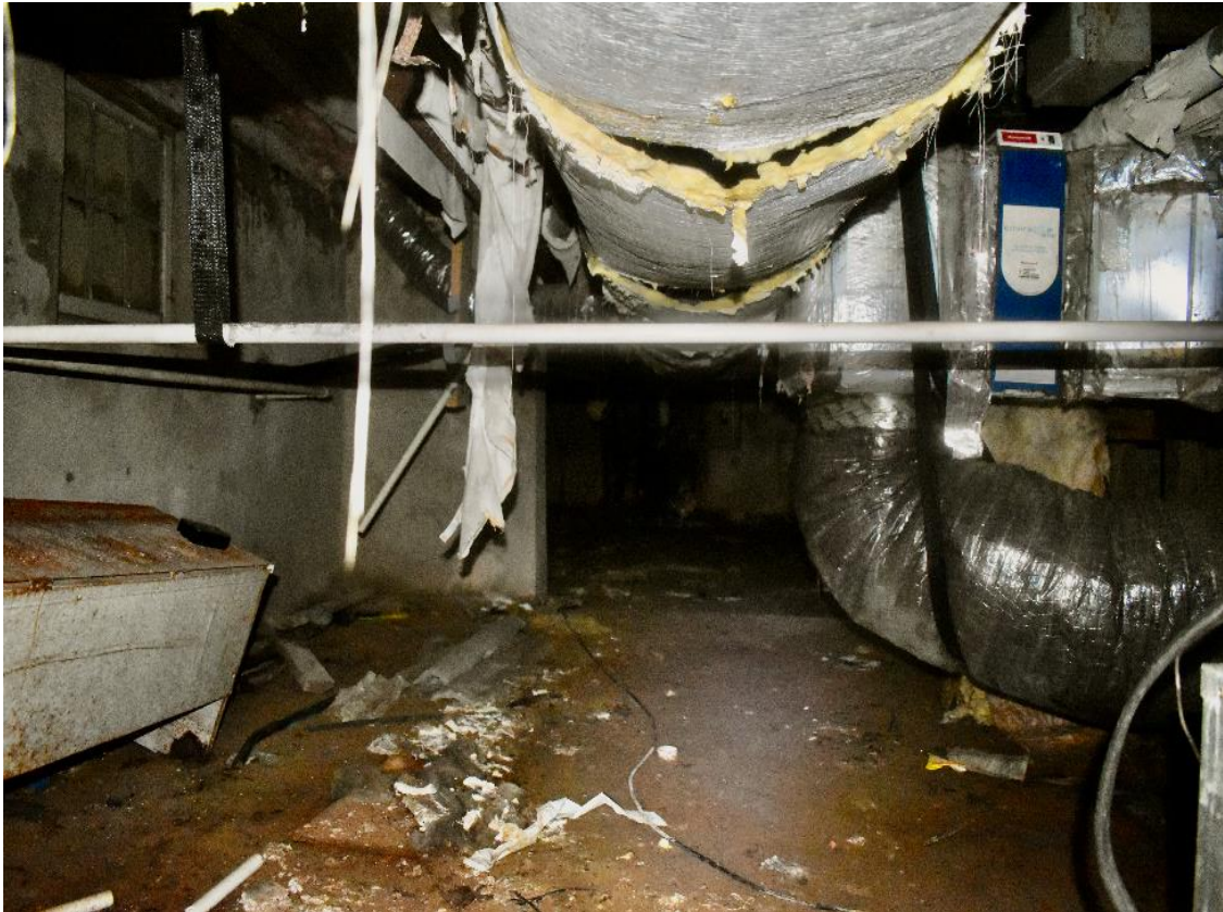
Fig. 27. Basement - note damp floor and damage to ductwork from high humidity levels
