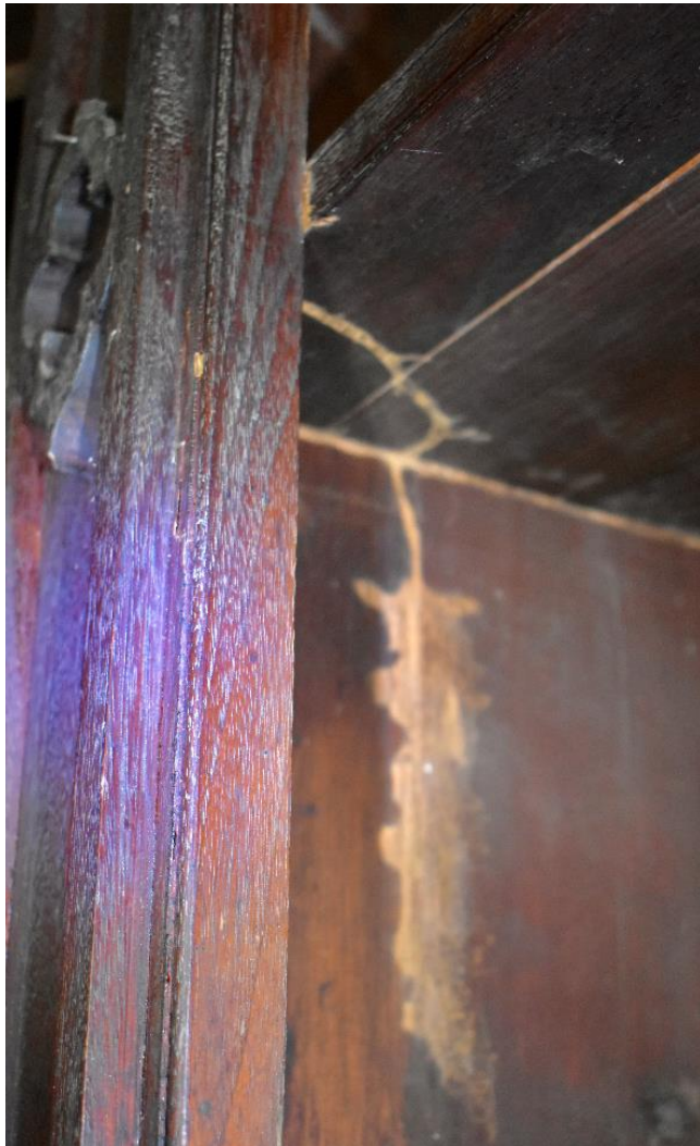
Fig.28, Termite damage inside a built-in bookcase in the library.
