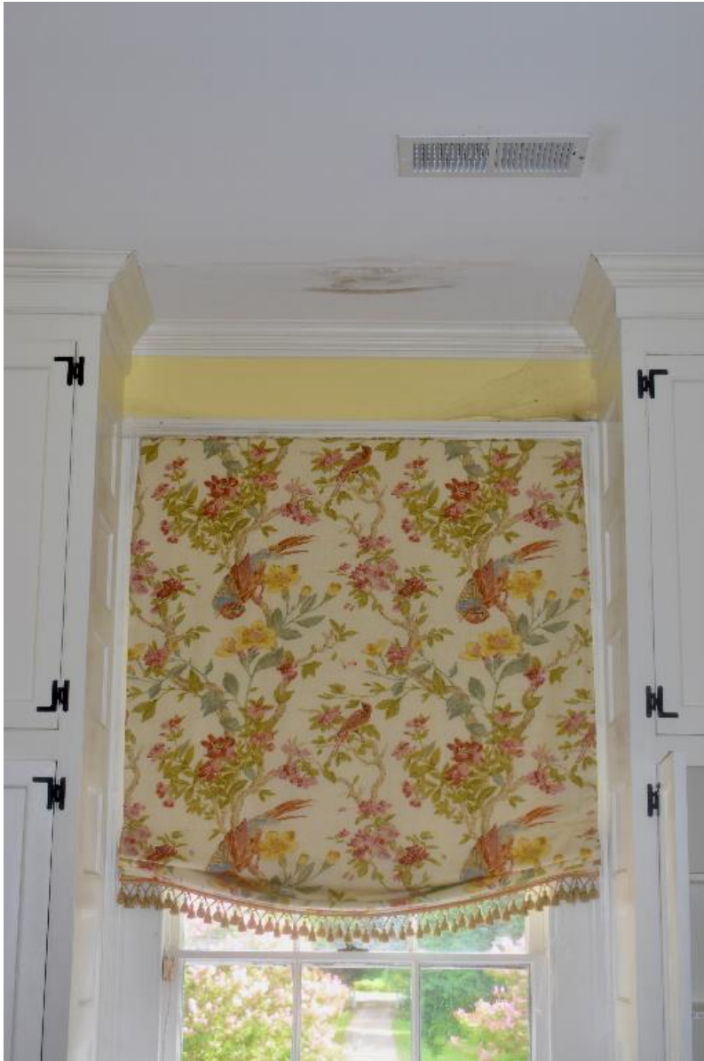
Fig. 19 Ceiling stain from active leak – second floor hallway – north end.
