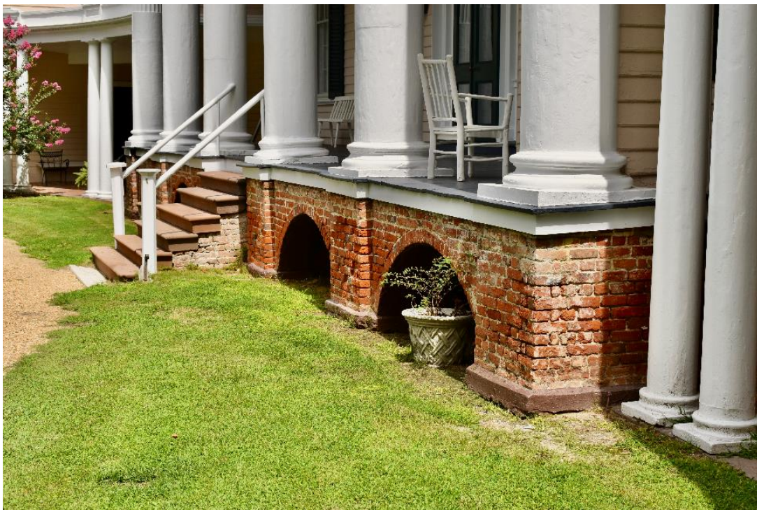
Fig. 25. Erosion at foundation of south porch.
