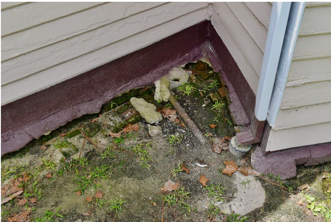
Fig. 23. Foundation erosion on the north elevation, west side
