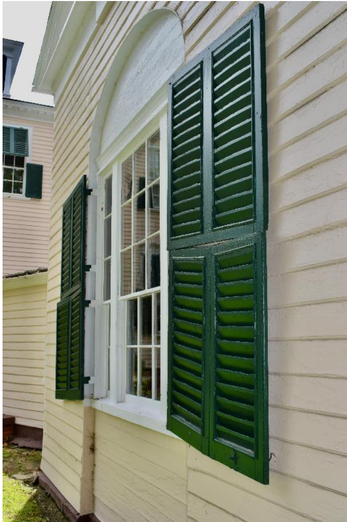
Fig. 29. North elevation, west wing - note sagging blinds.
