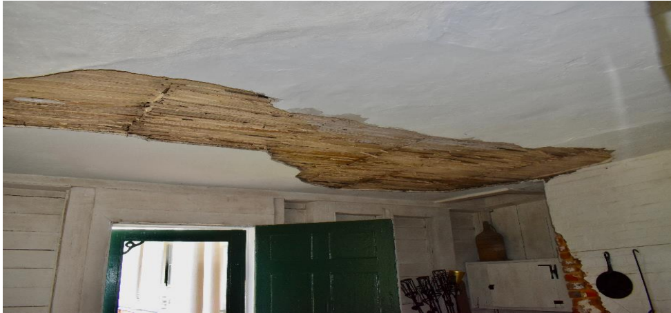
Fig. 13. Damaged and falling area of plaster in the original kitchen
