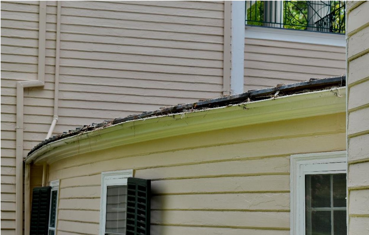
Fig. 22. West (north elevation) hyphen – note damaged and clogged gutter..
