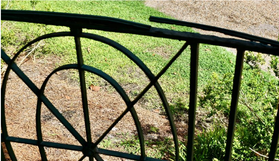
Fig. 12. Damage to original wrought iron porch railing
