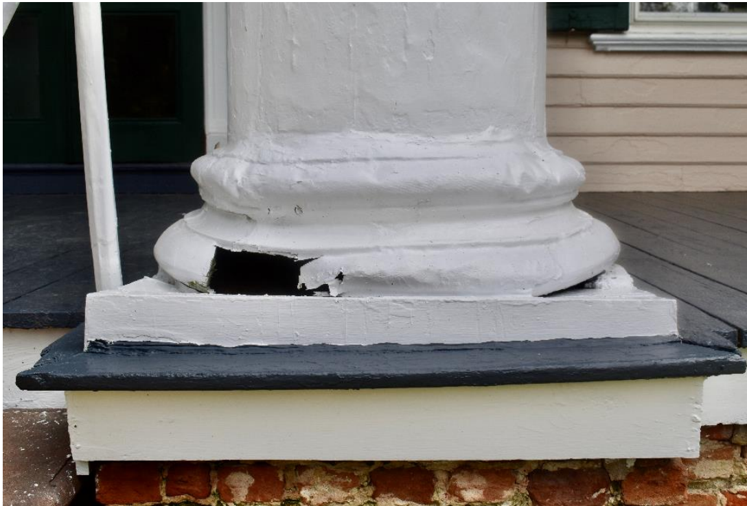
Fig. 15. Deteriorated column base – south porch
