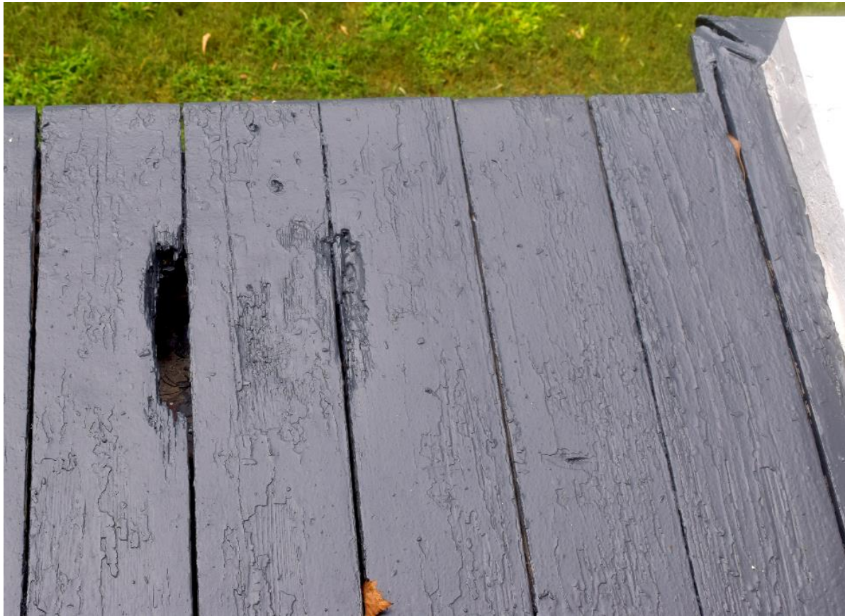
Fig. 16. South porch floor decay. Deterioration was also noted in areas of the outer porch framing member.
