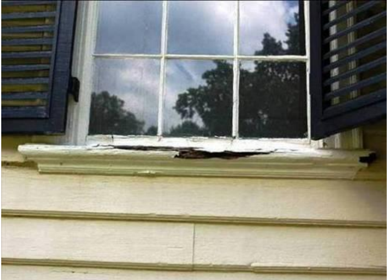
Fig. 4. Two-hundred-year-old windowsill decay, Sally Billy House, Halifax
