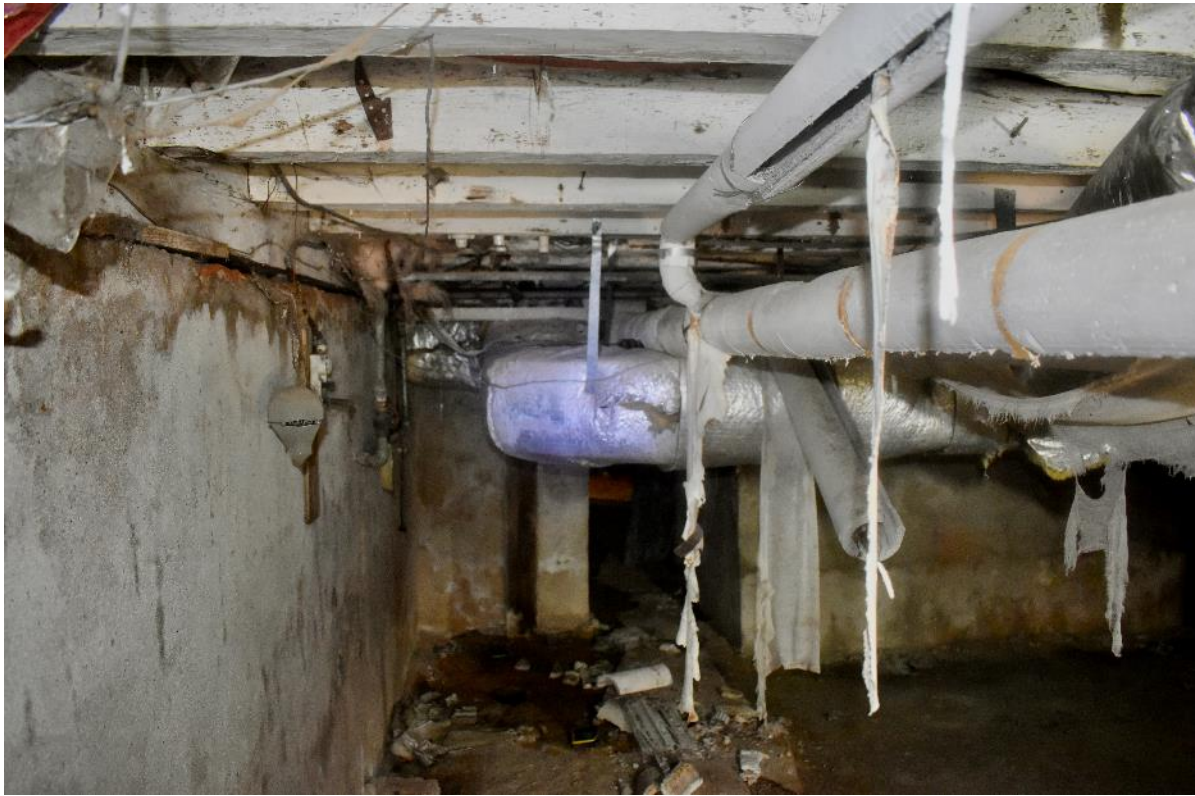
Fig. 5. Deteriorated pipe insulation in basement.
