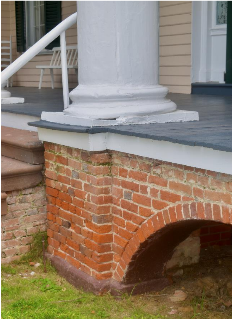
Fig. 17. South Porch – note deteriorated column plinth block and mortar loss.
