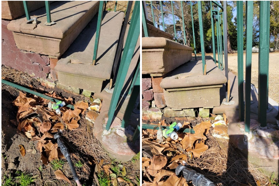
Figure 14 Bottom step cleaving on north stair and baluster missing with broken sets in stone
