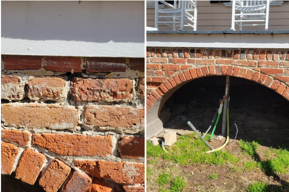
Figure 13 Mortar loss and bio-growth (left), Water pipe under arch (right)
