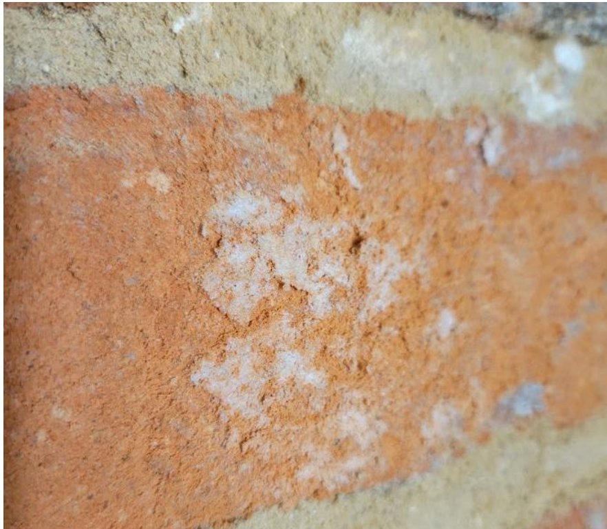
Figure 12 Salt efflorescence on the brick in the south room firebox
