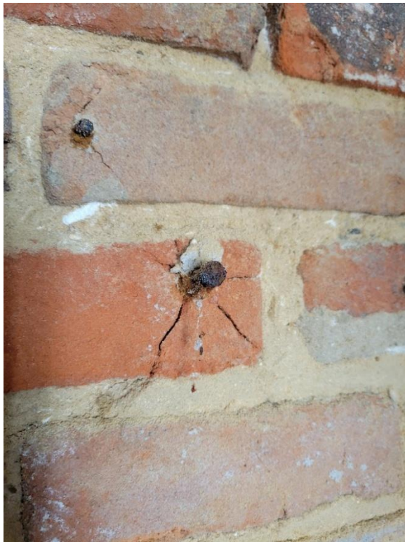
Figure 10 Nails within the bricks
