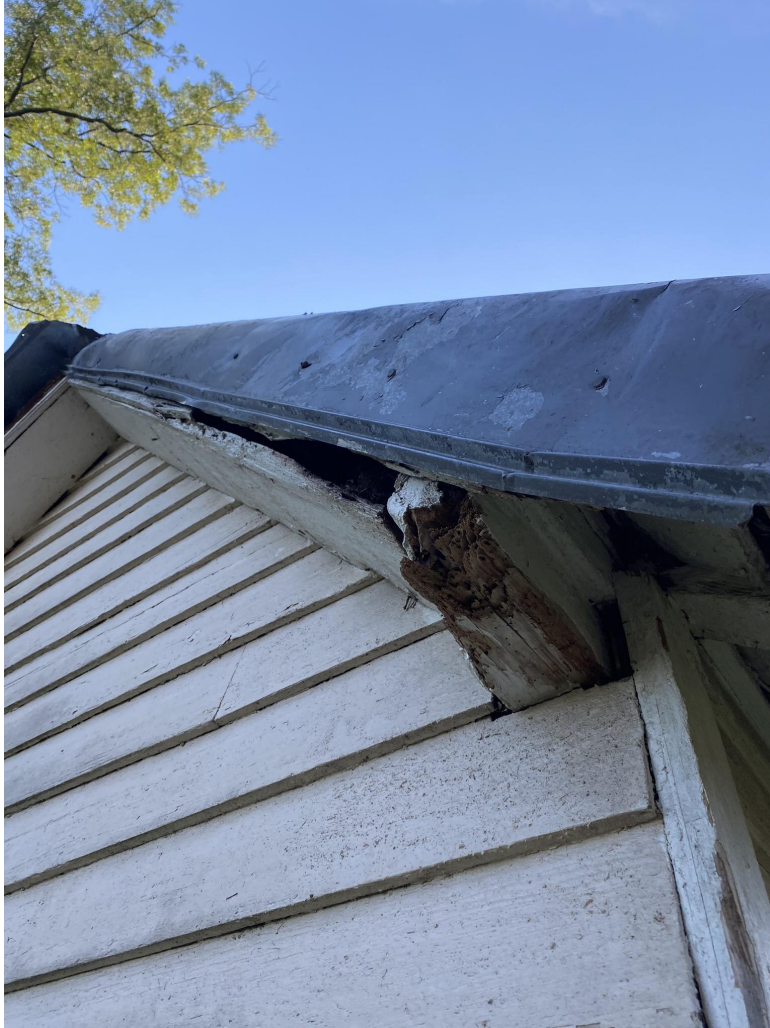
Rot and damage on rear cornice.
