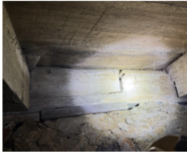
Fig. 30. Lap joint in south sill of c1719 core indicating a possible repair.
