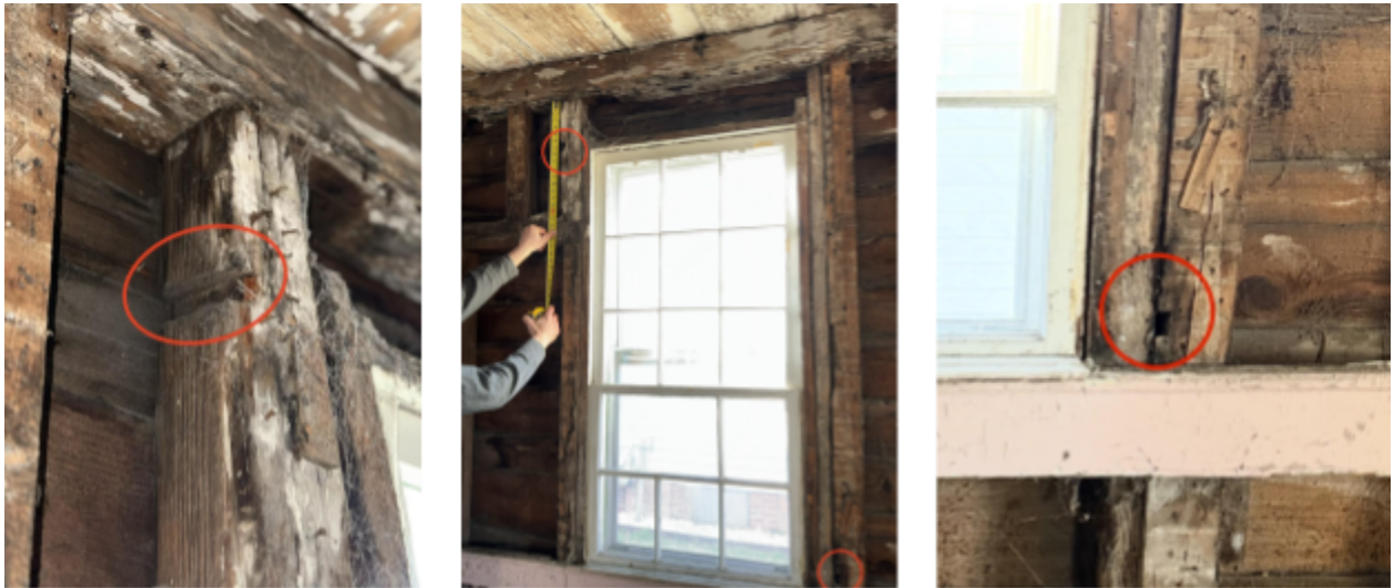
Fig. 19-21. Sill notches on west gable end for previous window, possibly an early modification using lap joints.
