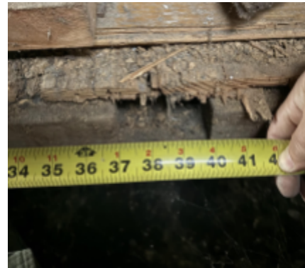
Fig. 9 Notches in shed room for trimmers spaced 37" wide. Note the sill appears to be replaced.
