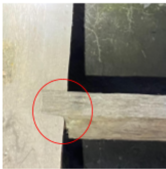
Fig. 7. Shed sill with joist notched with no pins.
