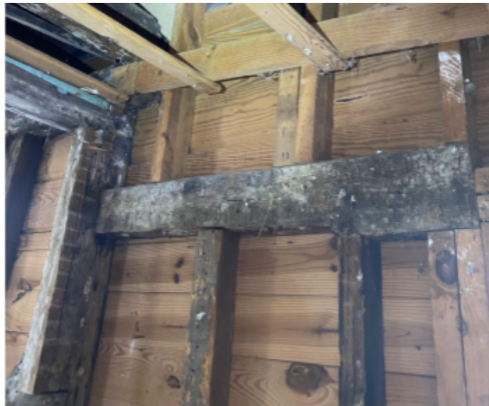
Fig. 32. Heavily modified header mortised into the south face of southeast corner post. Possibly part of an early shed modification.
