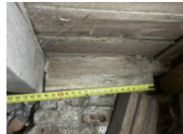
Fig. 4. C1719 trimmer and joist with notches indicating a firebox on the left side.
