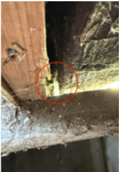
Fig. 16. Sill notch behind chair rail in south post of north window on east gable.
