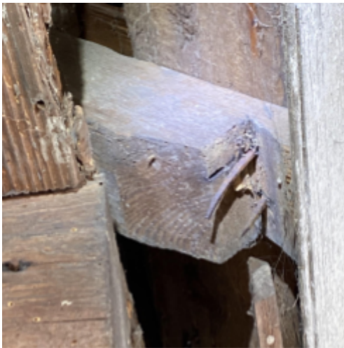
Fig. 34. c1719 notched rafter pulled out of the north false plate. Note wrought nails.
