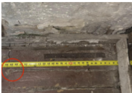
Fig. 5. Early fireplace evidence in flooring, south of chimney.
