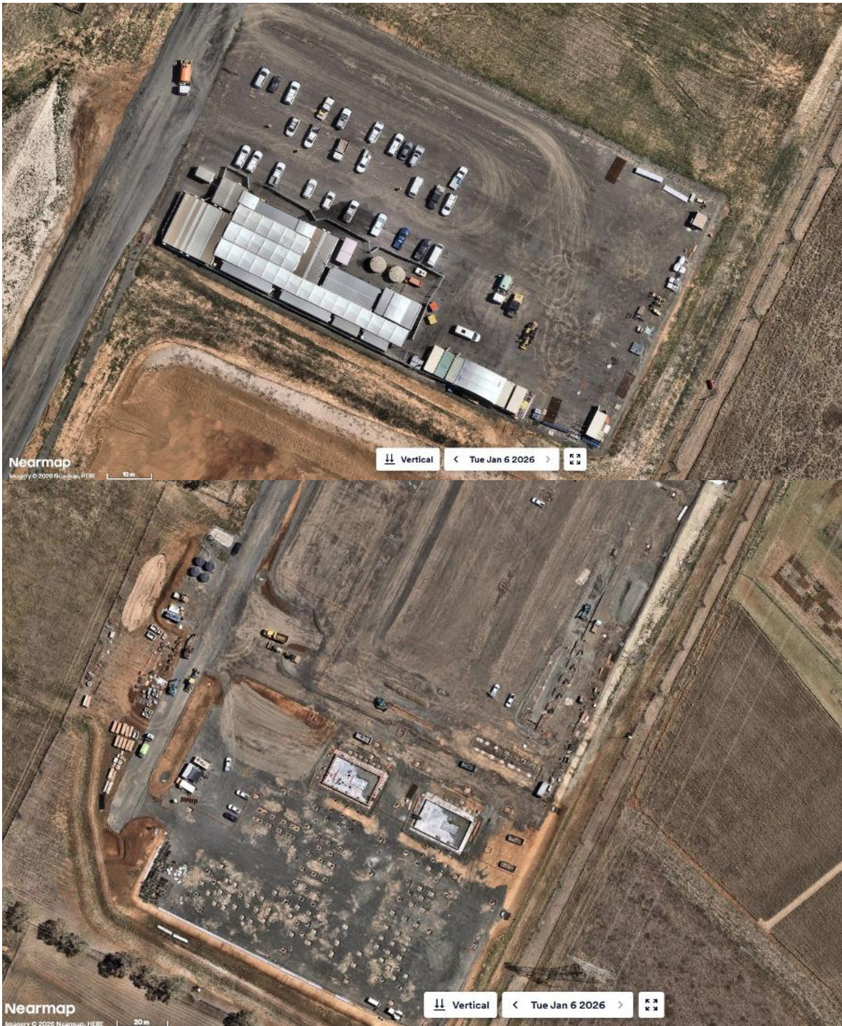
Photo B1-4: Aerial photograph of site carpark and BESS Construction site on 6 January 2026
