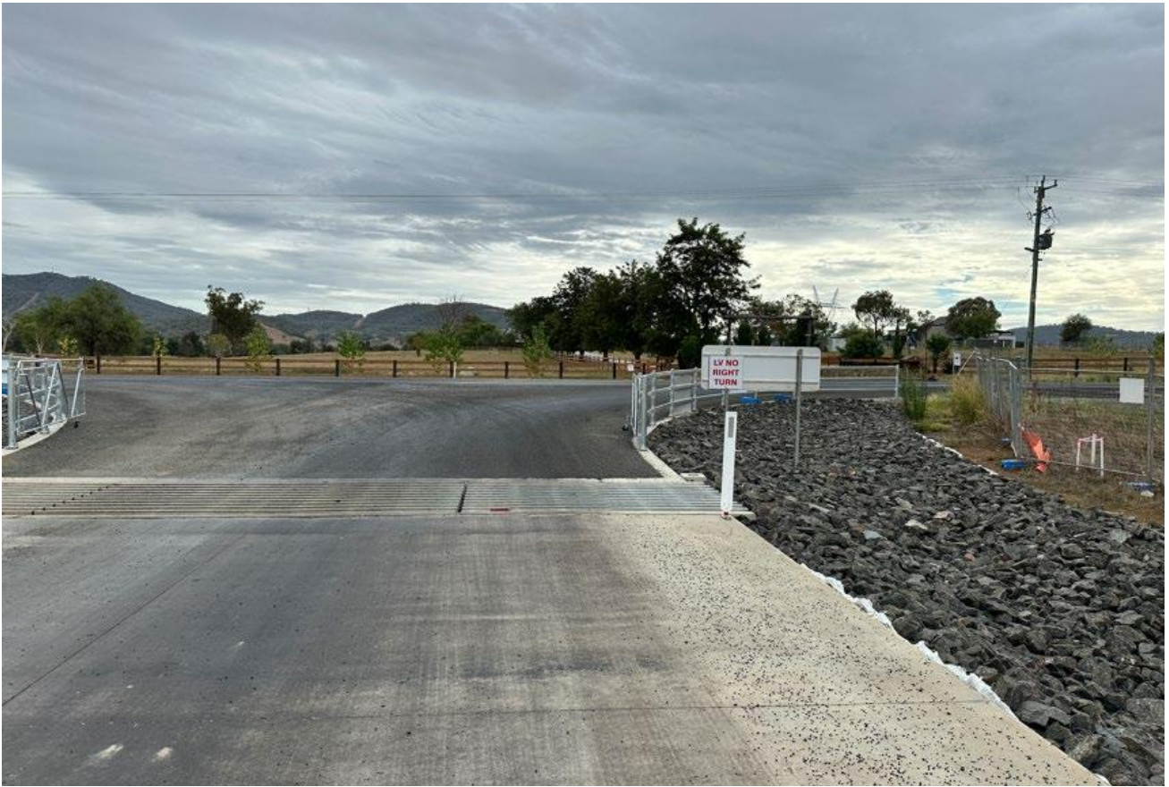
Photo B7-1: Road upgrade works at the site access point off Calala Lane completed
