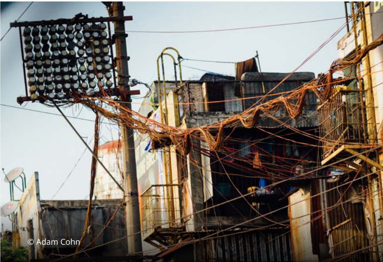
Informal electrical connections are a safety hazard, particularly in informal settlements where houses are built closely together with flammable materials.
