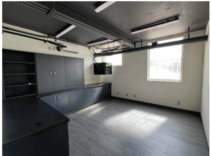
Manager's Equipment Room
