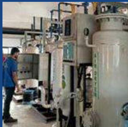
Desiccant air dryer
