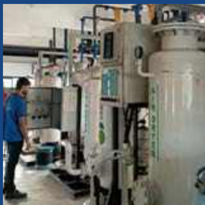
Desiccant air dryer
