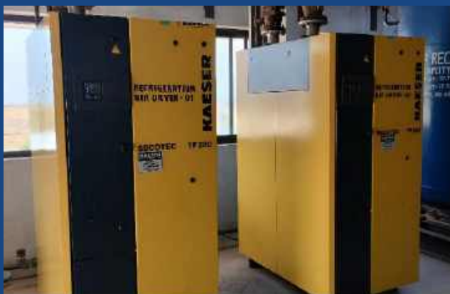
Refrigerant air dryer
