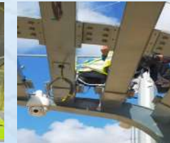
CCTV Video Surveillance System
