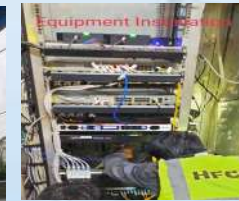
Fiber Optic Transmission System - FOTS
