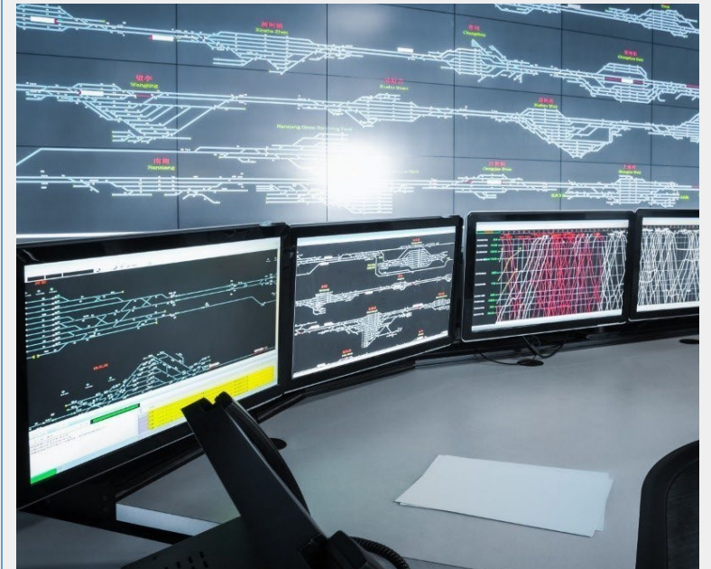
Implementing communication network including IP based Video surveillance system (VSS) for railways
