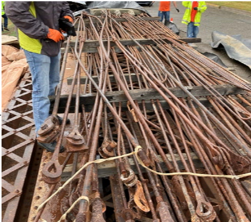
Figure 14: Lateral Bracing Rod Deformations
