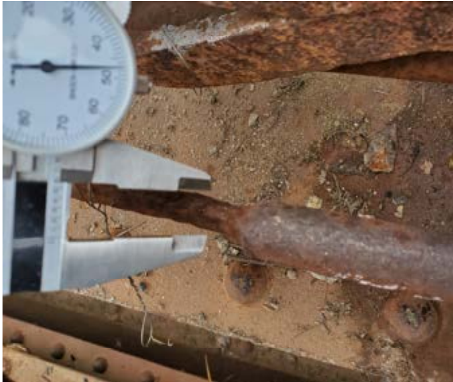
Figure 15: Major Rusting of Lateral Bracing Rods
