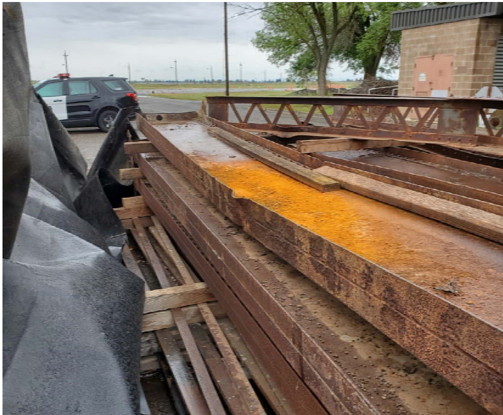
Figure 7: Rusty and Deformed Floor Beam Member
