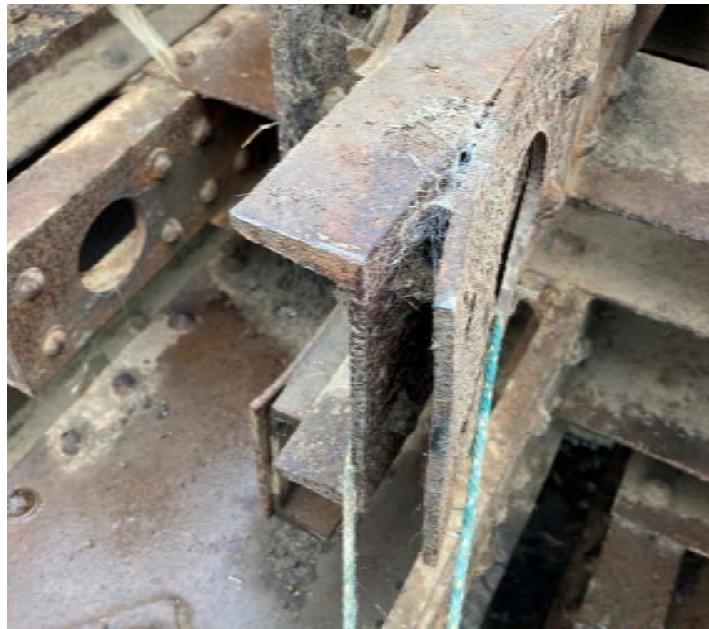
Figure 9: Diagonal Chord Web and Additional Plate Separation
