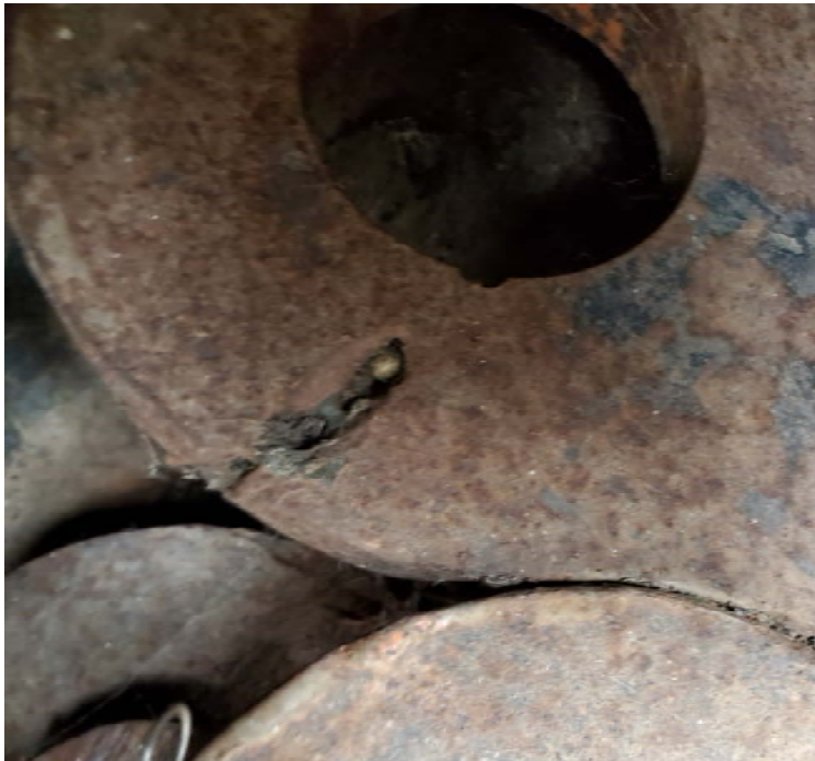
Figure 10: Damage in Straps and Bottom Chords
