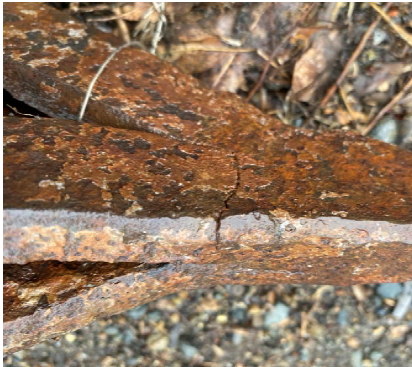
Figure 12: Cracks in Lateral Bracing Rods
