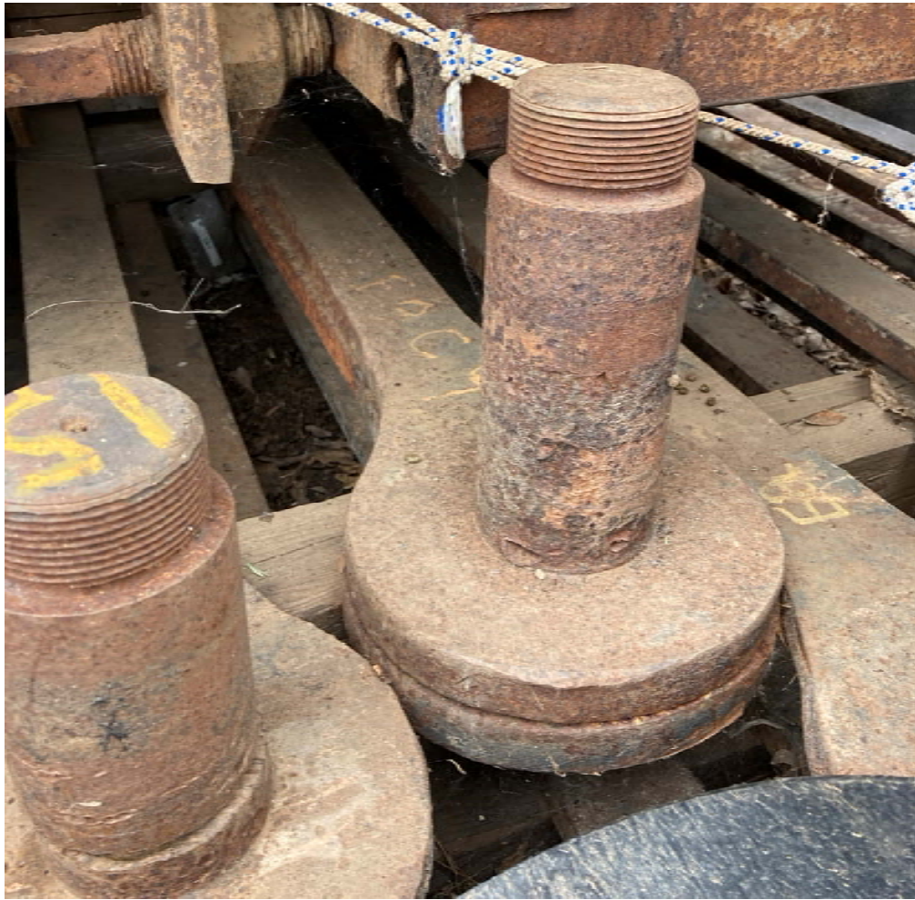
Figure 17: Cut Pin Connections Stuck in Members
