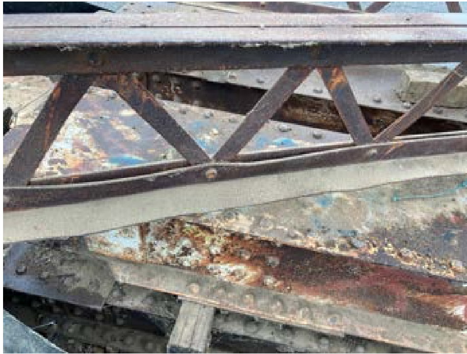
Figure 11: Portal Beam Flange Deformations
