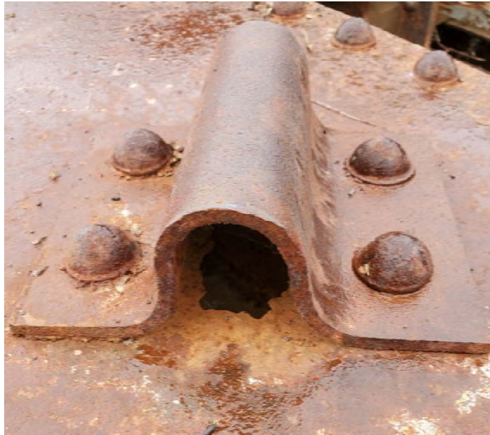
Figure 8: Hole in Top Truss Chord Plate
