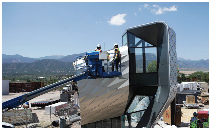
Top image: Not a single shingle on the USOM's façade had the same size or geometry
