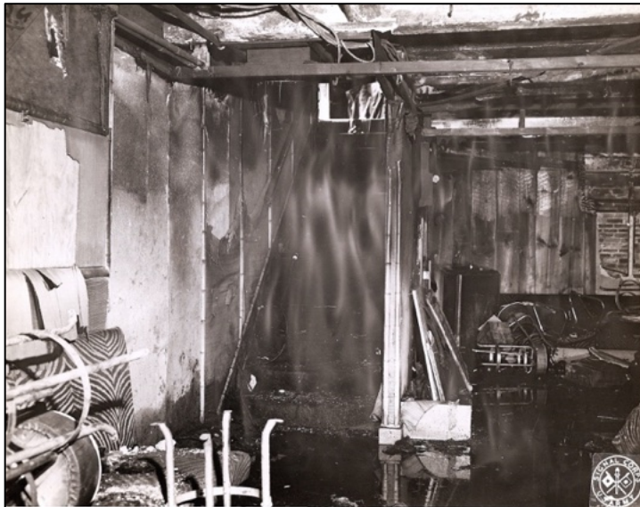
Melody Lounge, looking North, toward point of fire origin. (Boston Public Library)
