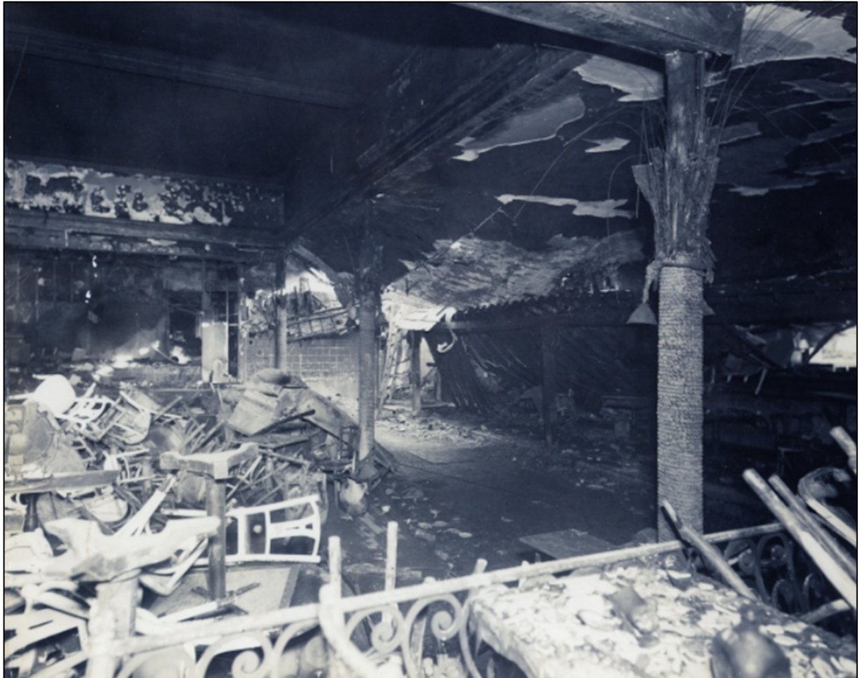
Main Dining Room, looking East toward Passageway to New Broadway Lounge, where fire damage was most intense and caused portion of roof to collapse. (Boston Public Library)
