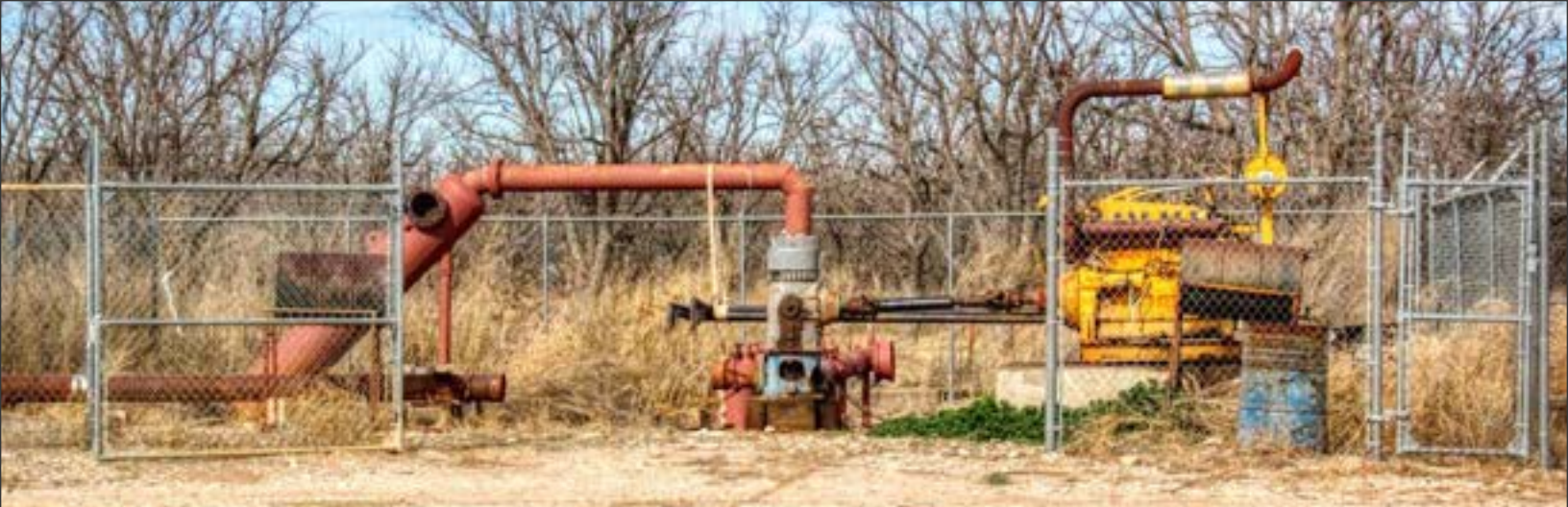
Water well with pump and engine in the Leon-Belding Irrigation Area with a pecan farm in the background (taken on January 12, 2020 by Robert Mace)
