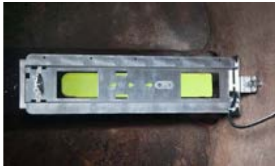
Installed Sensor Bracket on Wall Mount Bracket
