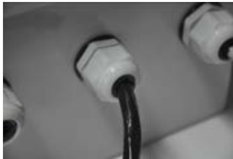
Monitor communication cable running through middle cable gland with plastic nut on XIO or XBUS
