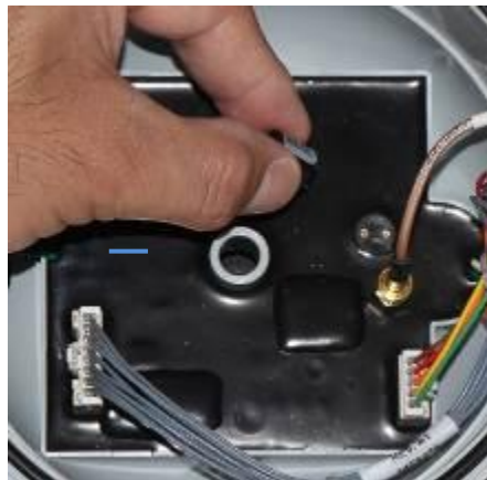
Blue fuse removed from the regulator board
