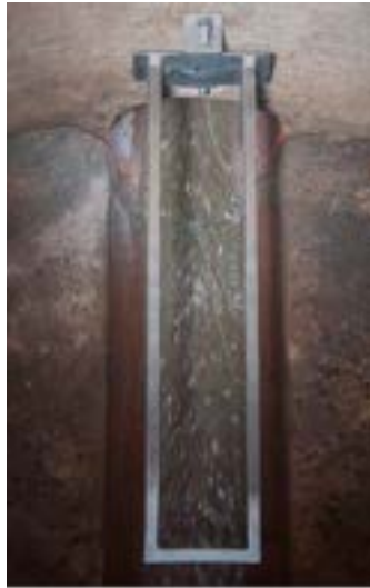
Installed ParaDepth/ParaFlow Wall Mount Bracket
