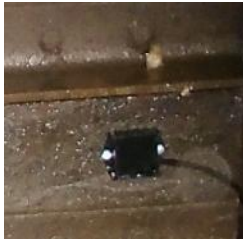
Inclinometer attached using Stainless Steel Screws
