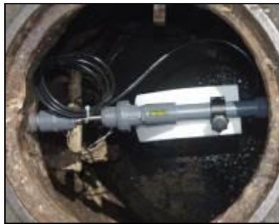
Long Range Sensor Fully Installed
