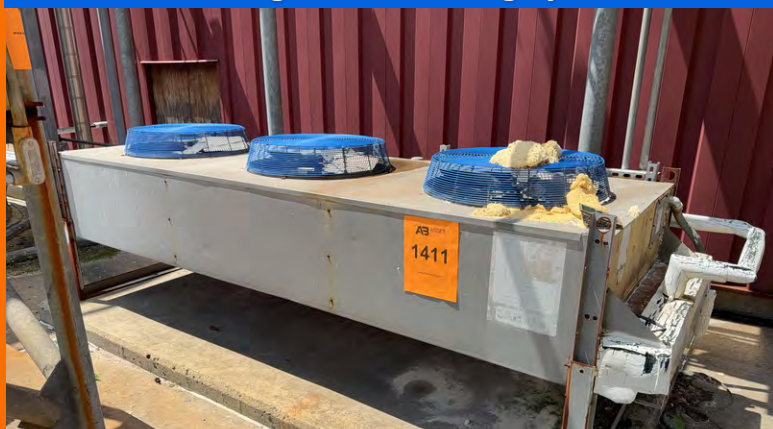
Compressed Air & Panel Cooling
