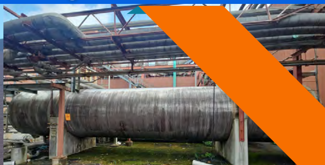
Gas, CO 2 & Utility Refrigerant Receivers
