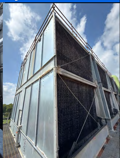
Utility Cooling Towers & Heat Rejection
