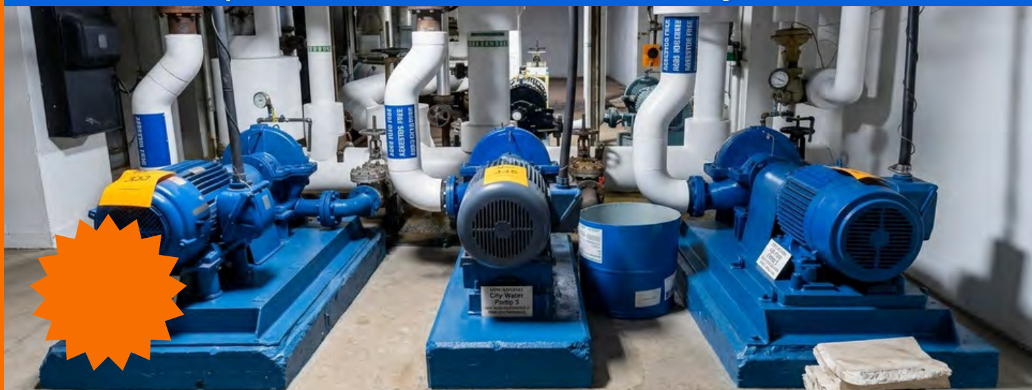
Sanitary Transfer & Yeast Recovery Pumps
