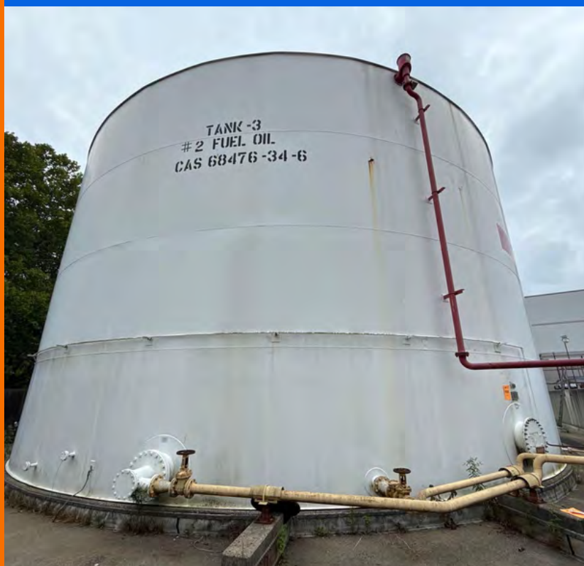
Chemical Storage & Containment Tanks (Corrosive-Rated)
