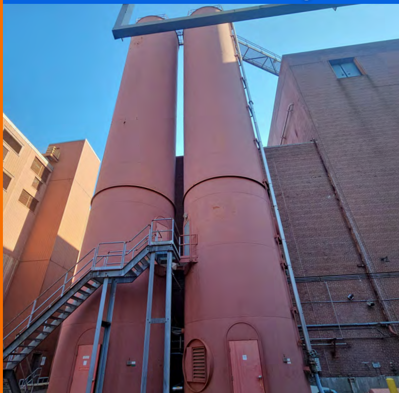
Raw Bulk Material & Product Silos
