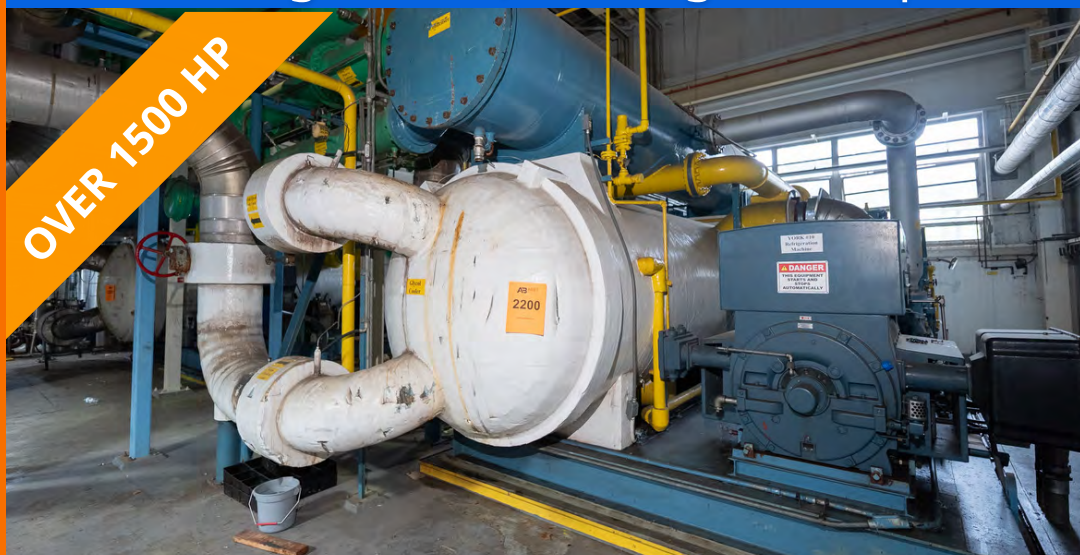
Process Chilling & Condensing Systems
