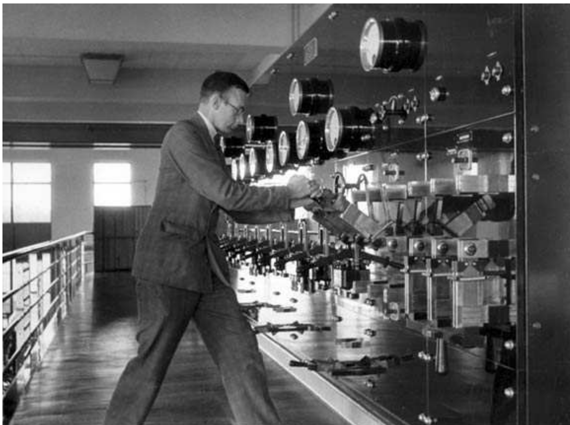
Droitwich 1935: Machine Room Switchboard Knife switches feeding 415v 3ph supplies to mercury arc rectifiers. The switches were changed over daily and the blades frequently felt to check for overheating!
