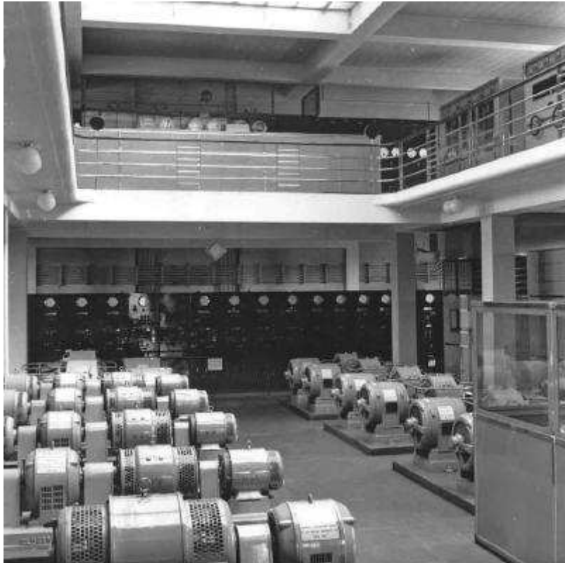
Droitwich: Lower transmitter hall showing filament, grid bias & aux.h.t. motor generators
