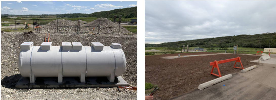
Figure 1 - Jokaso System at Pine Creek WWTP
