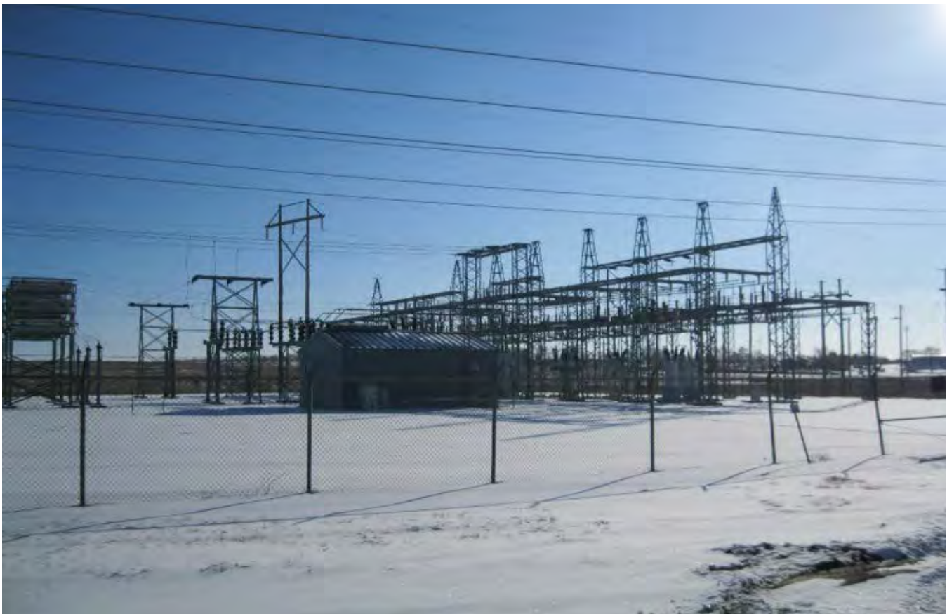
Figure 3.10: Example of electrical substation in the study area.
