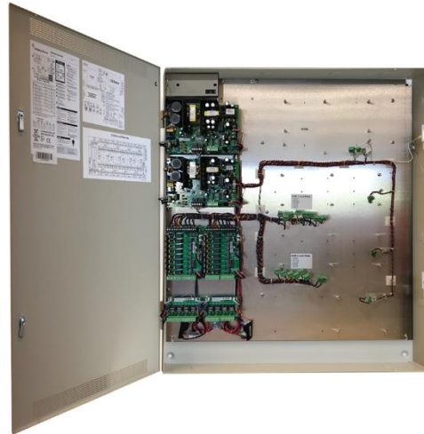
16-reader Ultra SE Wired System
