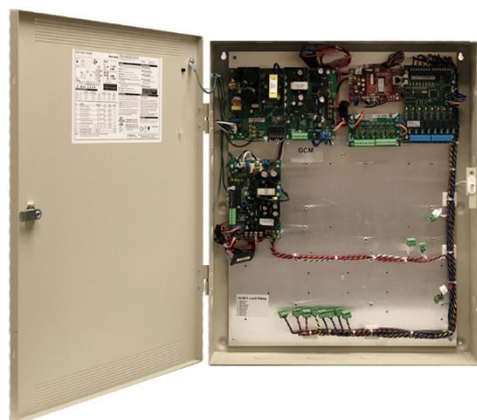
8-reader Ultra SE Wired System
