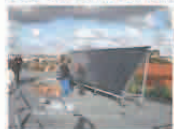
Chauffage solaire direct, crèche - Cherbourg (50)
