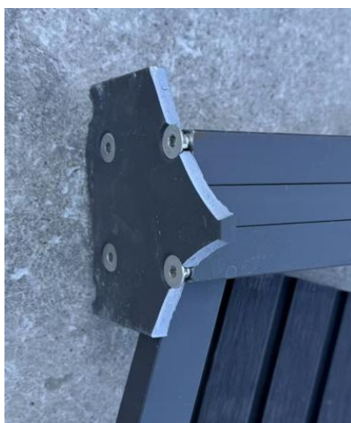
Photo 7. The fence specimen was damaged by the wind load at wind speed of 100 mph
