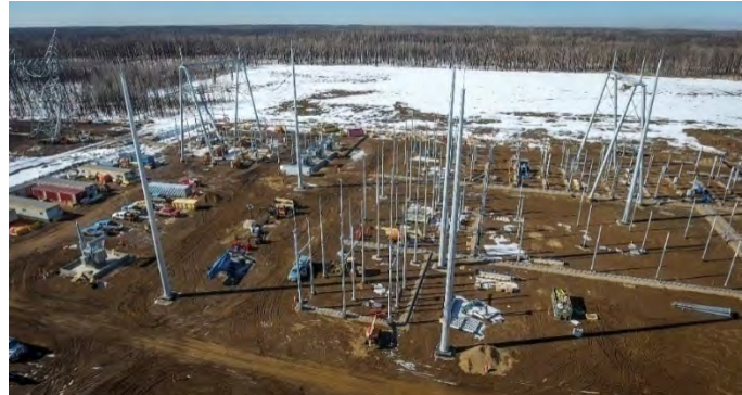
Figure 23: ATCO and Quanta combined our extensive electrical expertise and experience to develop a substation design for the Fort McMurray West 500 kV Transmission Project. This reliable substation is expected to exceed performance standards for many years.
