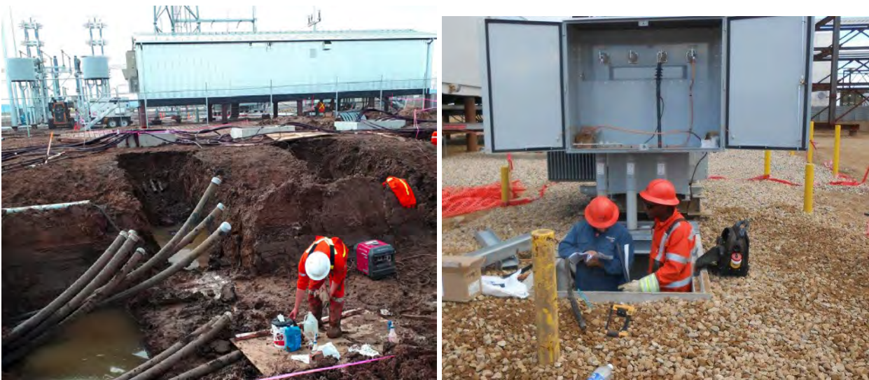
Figure 5: 25 kV three-phase underground feeders out of our Mowat Substation (left) and installing a pullbox and transformer at a customer site (right)
