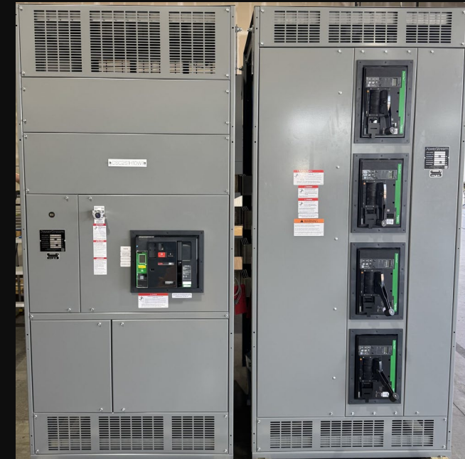
Semi Conductor Customer, Pre Fab Integration. 4000A Main Breaker with (4) 1000A feeder breakers, all rated at 100%. 84" Total Inches Wide.
