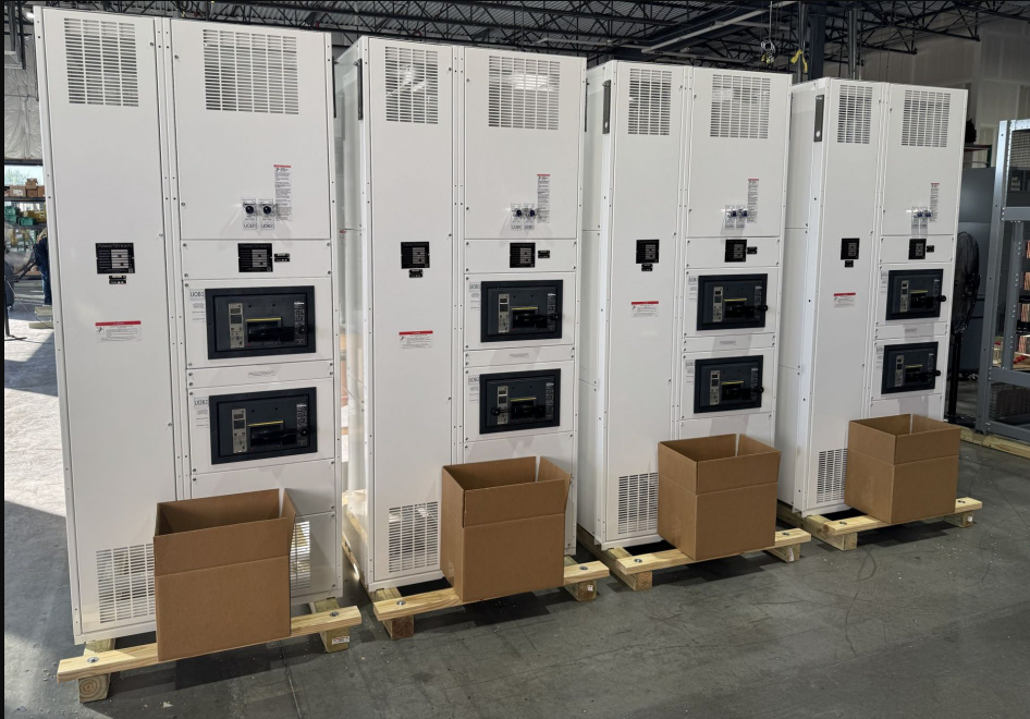
Four 750kVA UPS Output Switchboards
