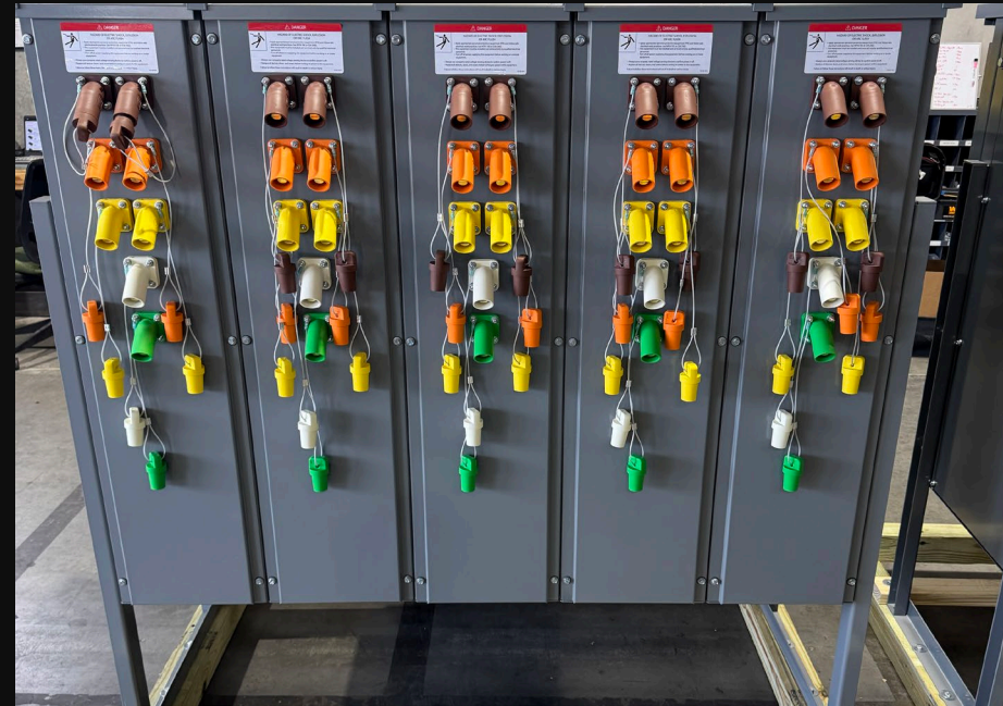
Modular Generator Combiner Boards
