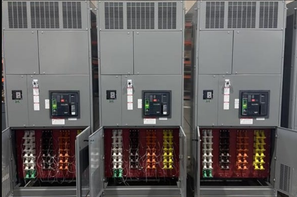
Switchboards with Integrated Camlock Connections
