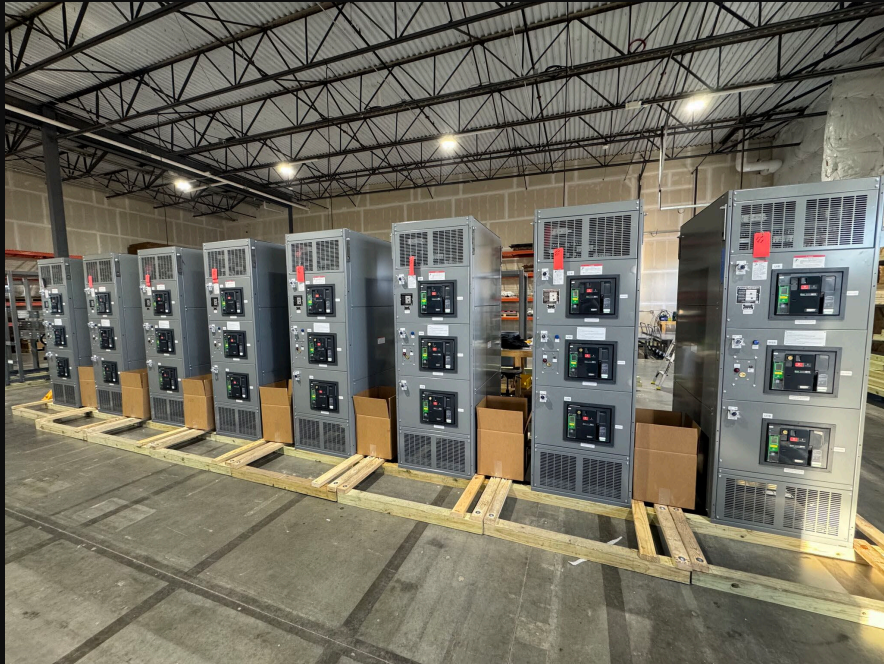
Eight 1.5 MW PowerPass Pro UPS bypass systems with Scheme 39 SKRU System
