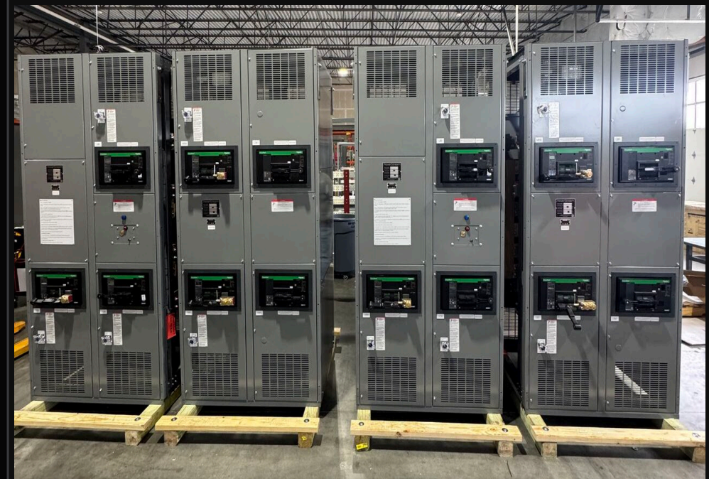
Two 750KVA Power Pass Tile Bypass Systems with Load Bank Breaker & Scheme 39 and 29 SKRU System
