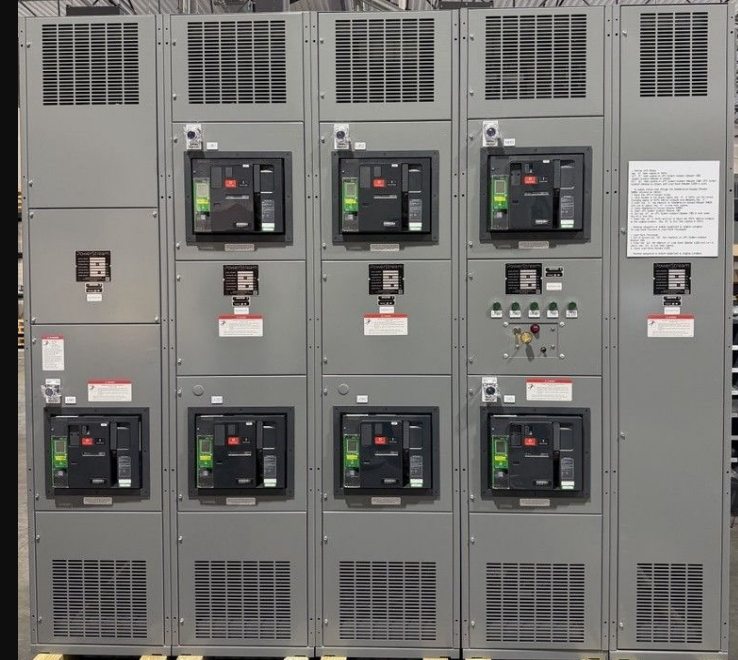
800kVA Dual UPS Power Pass Tile Board with Load Bank Breaker & Scheme 29 and 39 SKRU System
