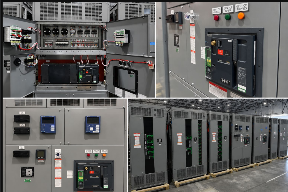
Hyperscale Data Center Customer. 4000A Main-Gen Switchboard with SELs, Power Quality Metering, UPS Backup, Surge Protection, IR window, & Fire Pump Section.
