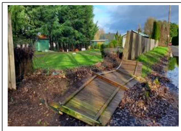
Wind Damage at the Front fence.
