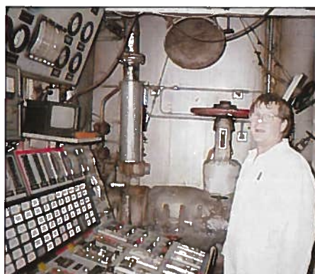
Chief Engineer Bill Smith on the Matson ship KAUIA at the control flat for the steam boilers.
