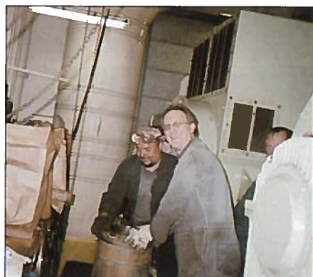
On the APL THAILAND are 2nd A/E Henry Faulhaber (glasses) and P.R.O. Bill Moreno. The two are in the process of removing a cylinder and rebuilding the generator.
