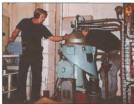
Aboard the SEALAND PRIDE, 1st A/E Scott Manchester is holding the purifier motor while 3rd A/E Bryant Salvesen sets up to put it in place. This photo is taken in the booster engine room in the main deck garage area.
