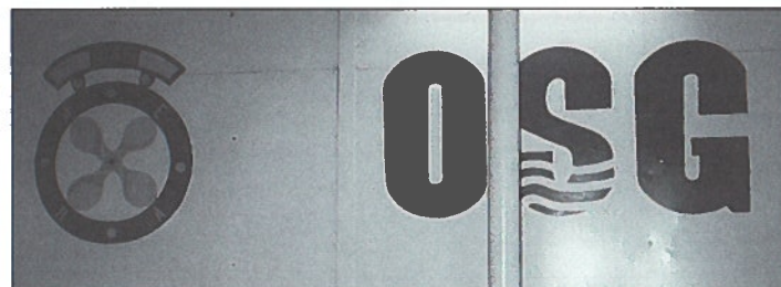
Engine room of the OVERSEAS NEW ORLEANS, covered under the OSG contract.
