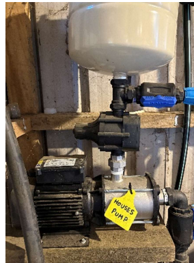
Existing Pump Set-Up
