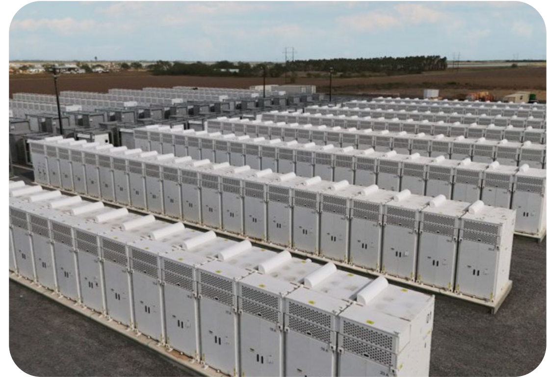
Apex's Great Kiskadee Storage facility in Hidalgo Co., TX.
