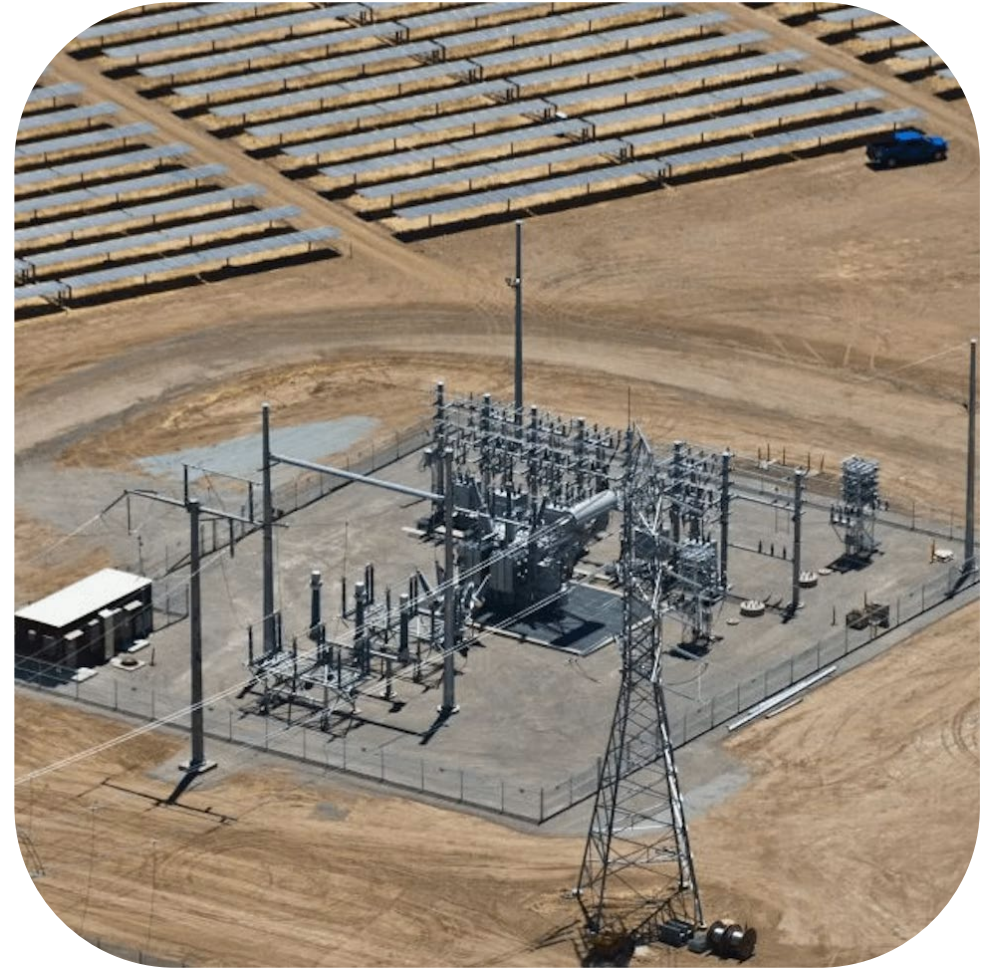
Example of project substation.
