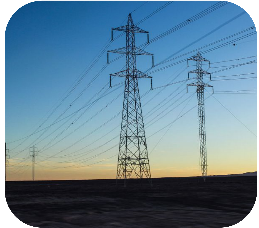
Example of overhead transmission line.
